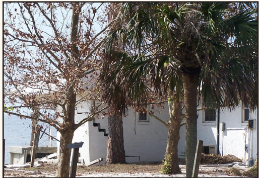
Figure 5-2: Structural damage to a concrete home (Source: Rosalyn Kilcollins)
