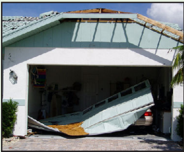
Figure 4-12: Because of their width, double-wide garage doors are more susceptible to wind damage than single doors. 19 (Source: Florida Hurricane Depot)
