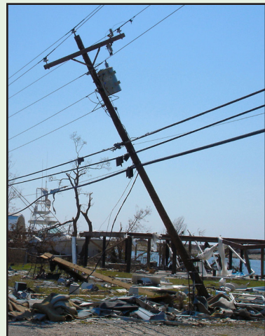
Figure 4-25: Downed or damaged power lines in a residential area can pose a serious danger to public safety. (Source: U.S. EPA)
